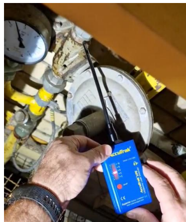
Figure 7 – The detection of gas leaks at the pressure regulator connection "UNIS" 1892 b
