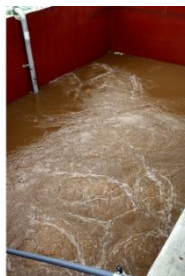
Figure 5 Denitrification tank (source: author archives)
